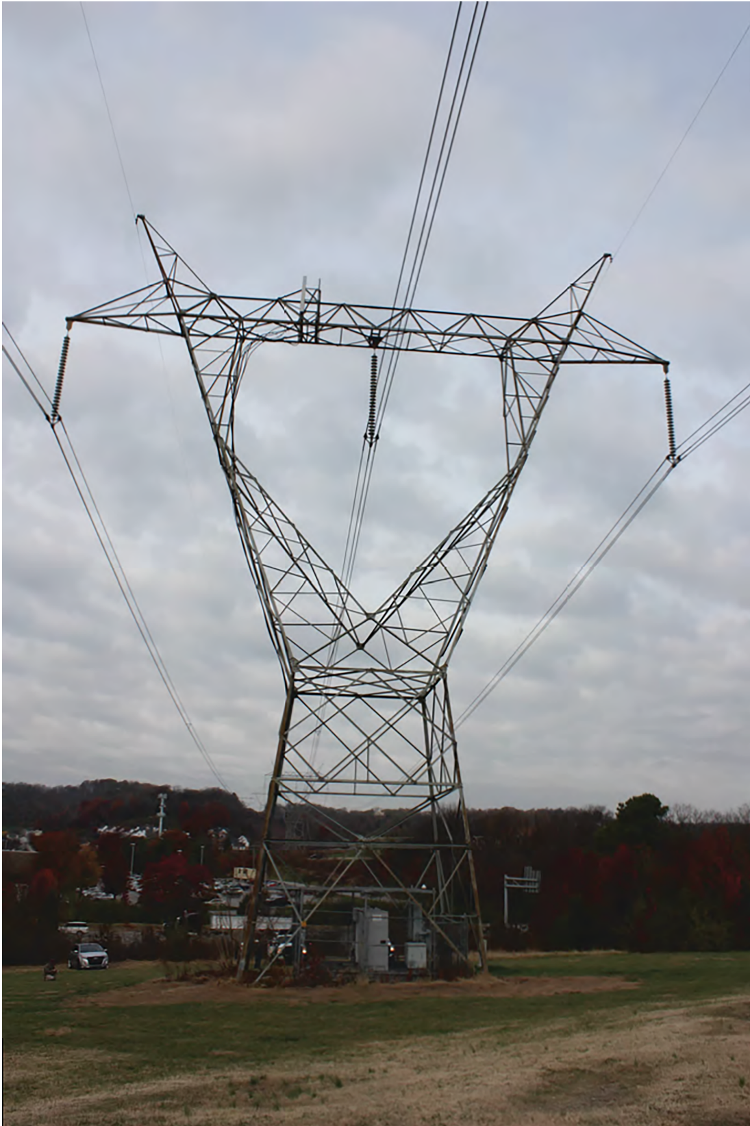
Figure 3.7-5. Typical TVA 500 kV Structure
