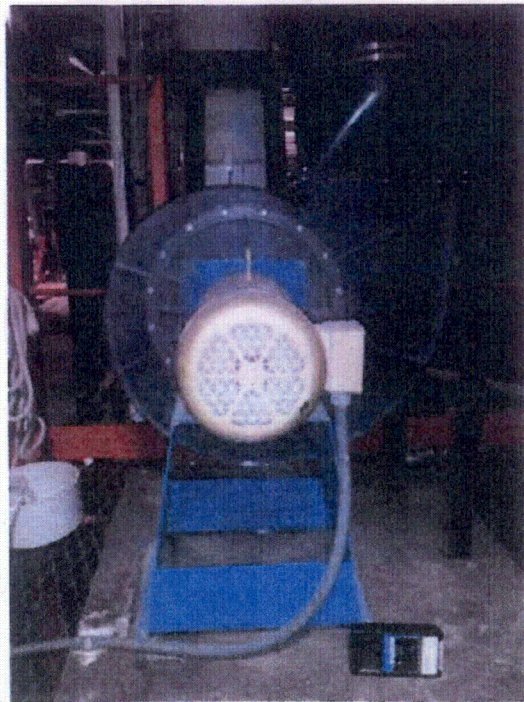
#7 Chemical Mix Tank Demister
