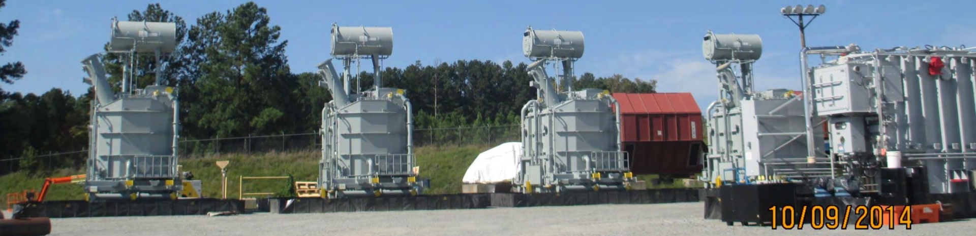
Unit 2 Main & Auxiliary Transformers
