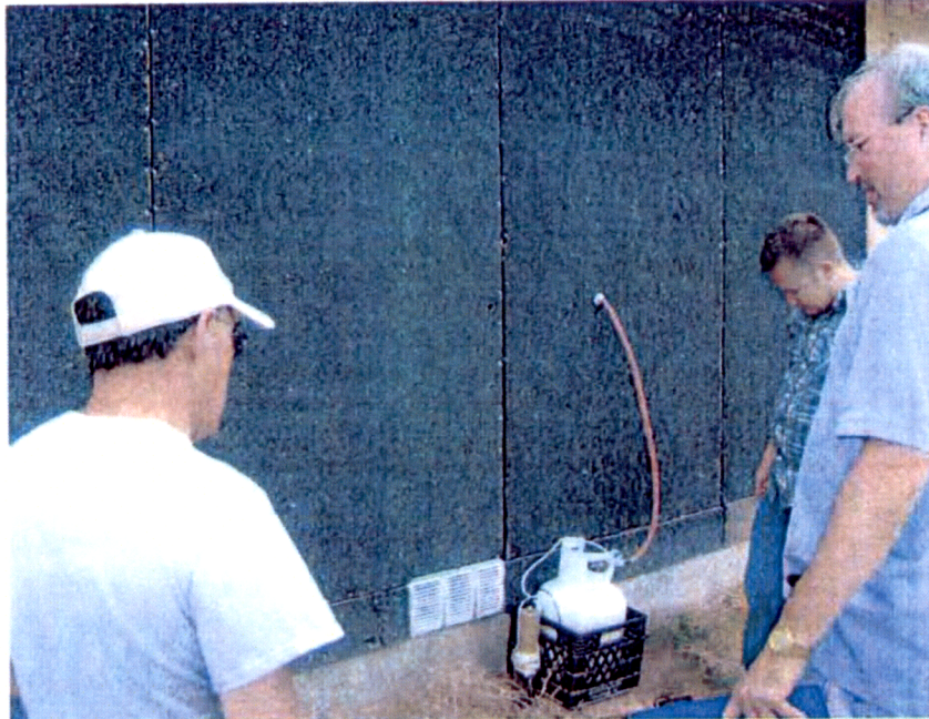
Photo 3: The “hot” propane tank attached to the building.
