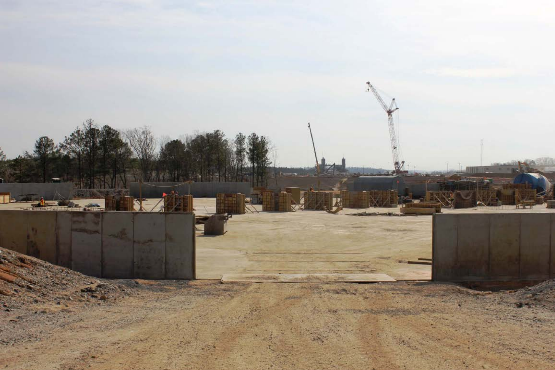
02. 09.12 Cooling Tower 2A
