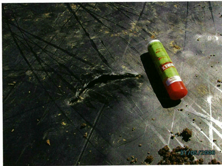
Fig. A.53. Close-up of unintentional hole from installation found via geophysical investigation.
