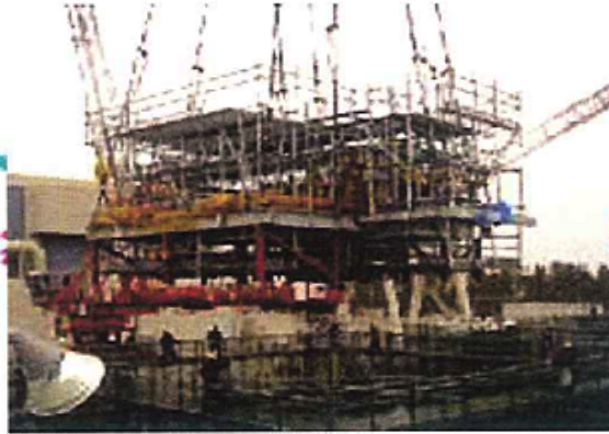
Piping Unit in T-G Pedestal Module
