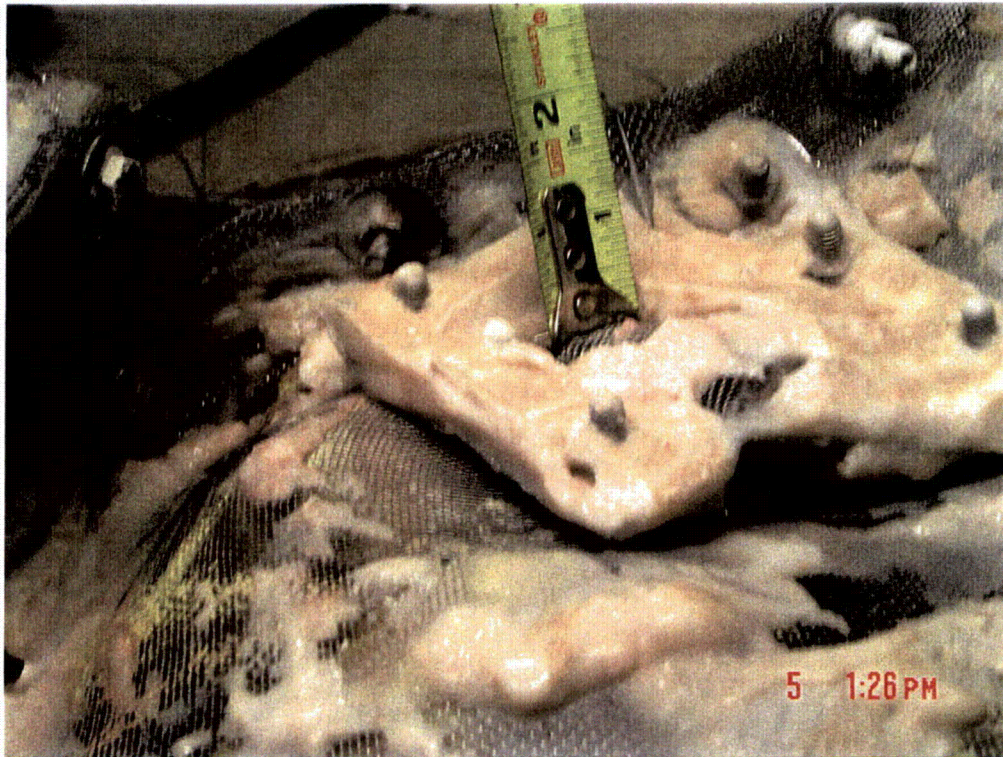
Figure 4-184. Stainless steel mesh covered with gel-like material.
