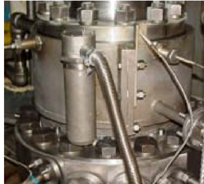
RCP Seal Standpipe
