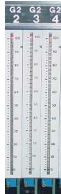
Control Rod position indicator
