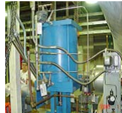
Valve after Engineering Change Package
