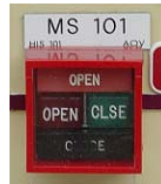
MS101 Control Room indicator
